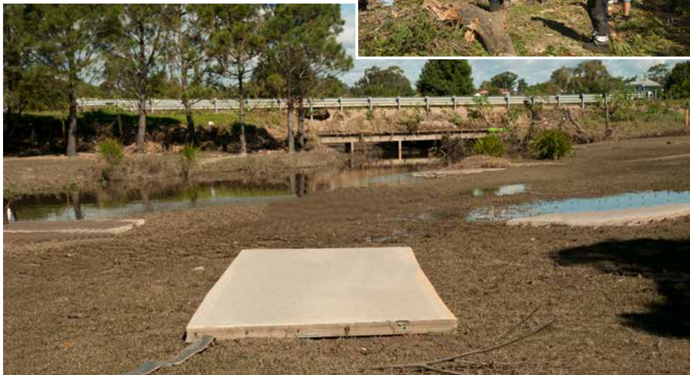
18th Fairway at 2 Mile Creek with cart path washed away, 2015
